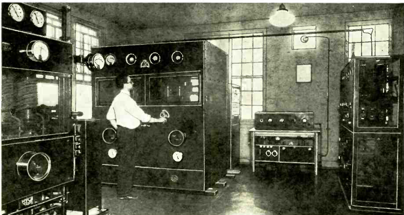
View of power amplifier unit at W3XAL, the National Broadcasting Company's station located at Bound Brook, N. J. (Fig. 2.)
